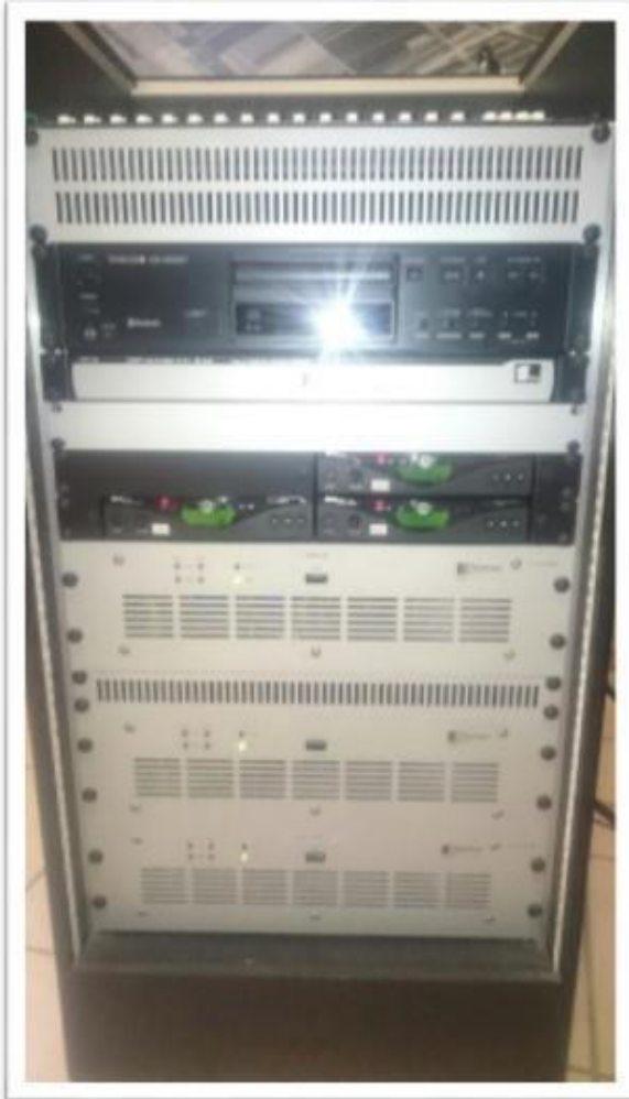
Mobiles Rack Front
